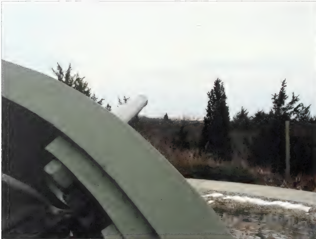
Figure 5.11. View east from south gun platform, Battery Gunnison. The downrange views from gun emplacements and battery commander's stations are significant to the historic operation of the batteries and should be reestablished to greatest extent practicable. The evergreens located closest to the gun in this image are growing upon the engineered slope. Once these have been removed, downrange water views can be evaluated and in limited instances tall, individual woody vegetation removed on a case-by-case basis (Olmsted Center, January 2009).
